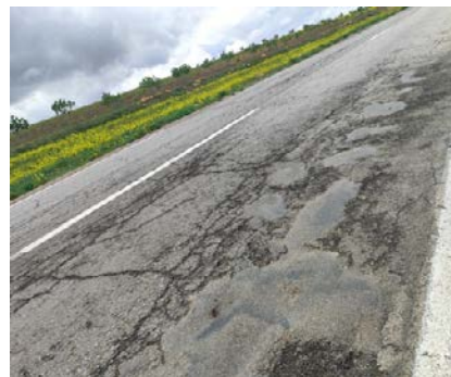
Figure 5 – Slight rutting indicating initial surface deformation
