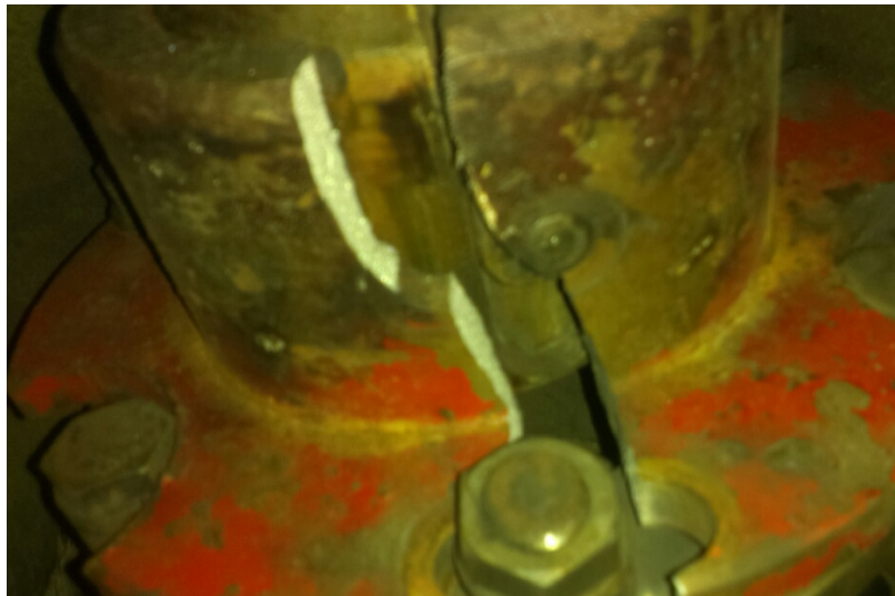
Figure 3 – Broken flange of the elastic coupling on the mini hydro generator flywheel
