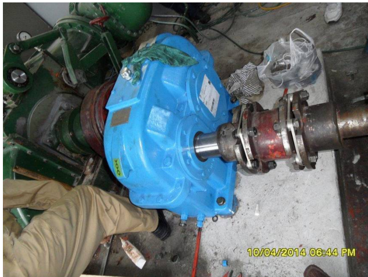
Figure 5 – Display of the assembled ARPEX couplings on the multiplier of the hydro power plant
